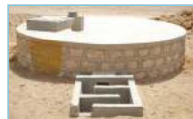
Rain water harvesting
